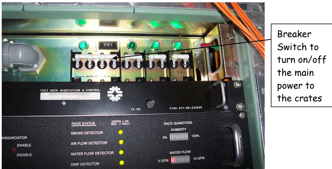
Figure 2) Breaker switch on each rack to use to turn on/off the main power to the racks.
